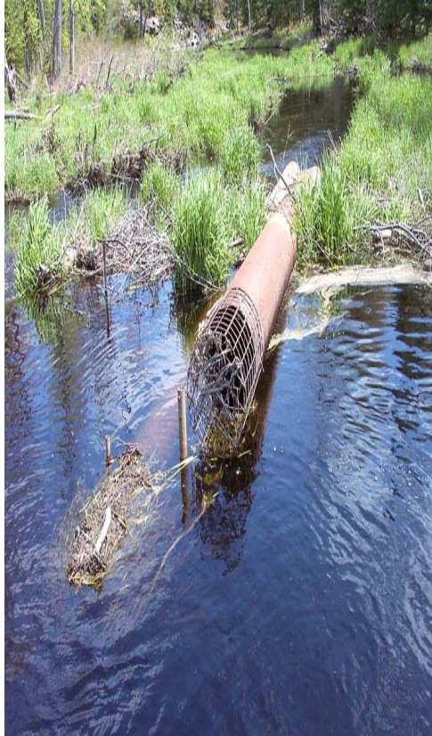
Damaged Beaver Baffle
